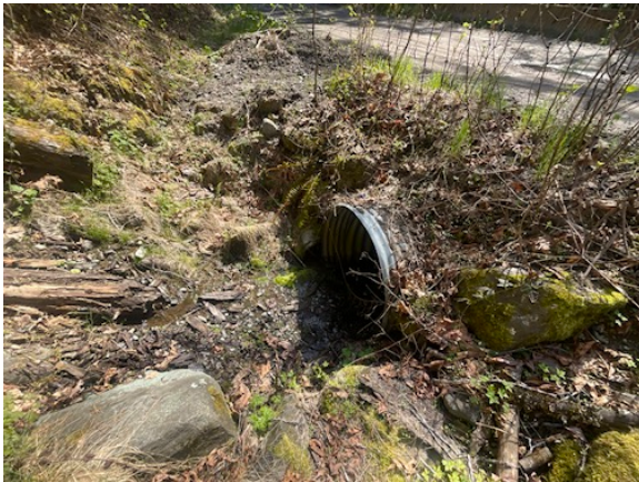
Inlet maintenance required
